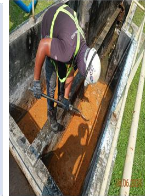
Sewerage Treatment Plant Maintenance
